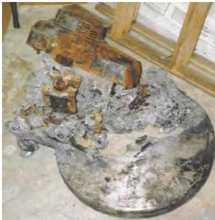
Figure 12.1 Melted machine deck after fire in school building
